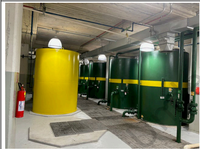
Photo 52: Oli-water separators on lowest floor of powerhouse
