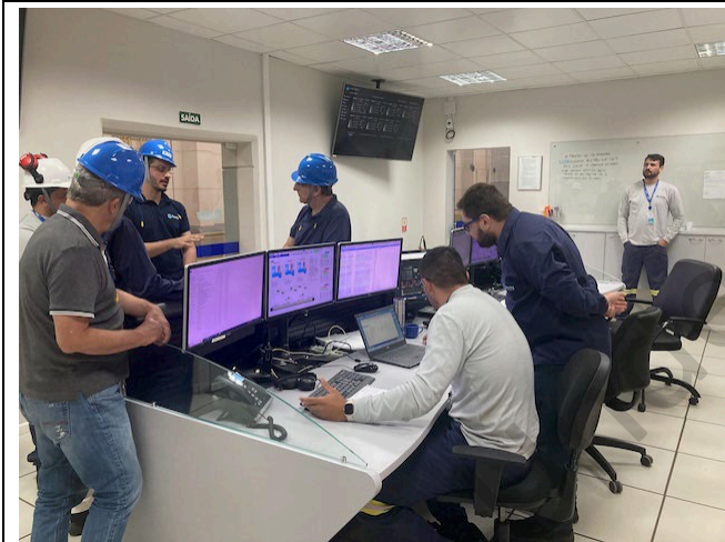
Photo 34: Powerhouse control room
