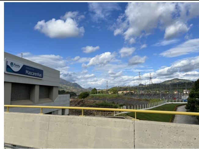
Photo 25: Short transmission line to substation
