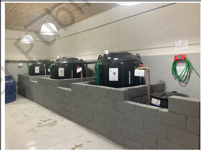
Photo 53: Sewage treatment on lowest floor of powerhouse
