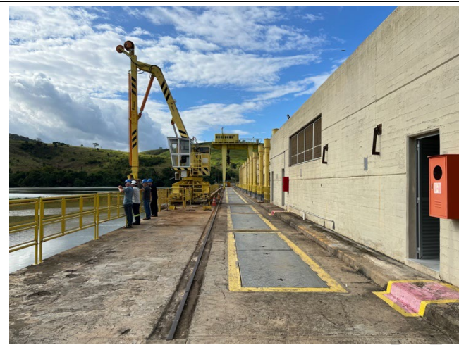
Photo 28: Upstream trash rack cleaning equipment
