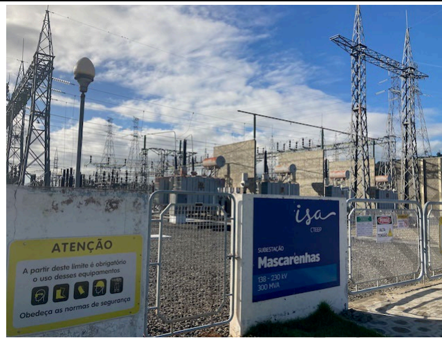
Photo 26: ISA CTEEP substation at Mascarenhas HPP
