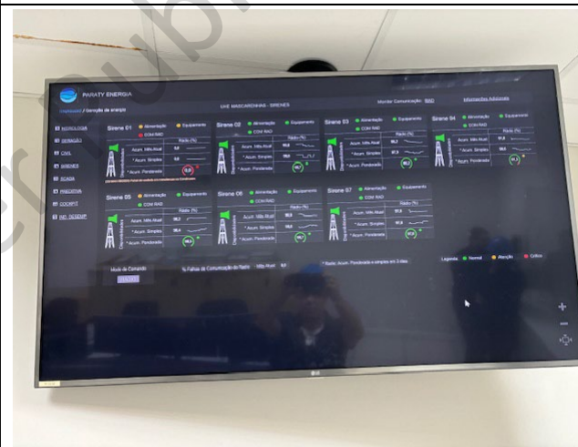
Photo 41: Operational status of the warning sirens
